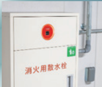
Piping parts for fire extinguishers
